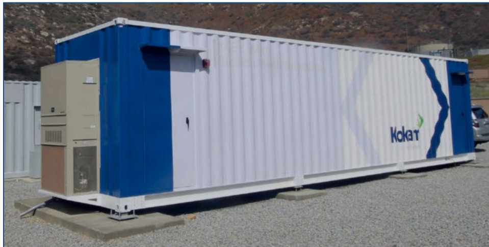
Kokam 40' Containter BESS
