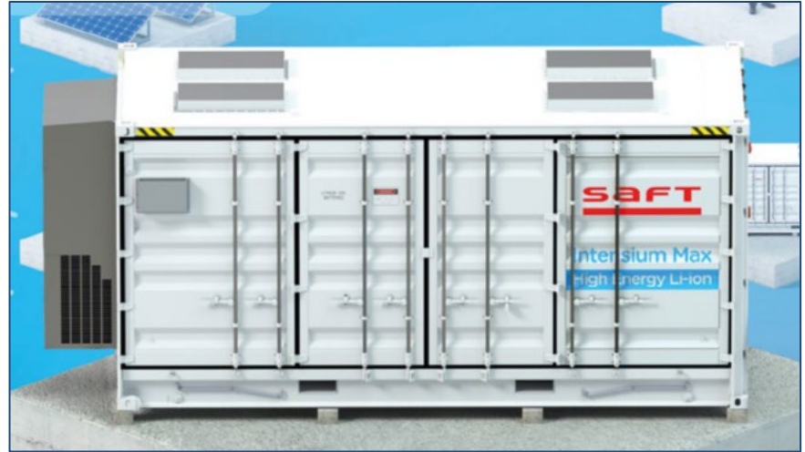
SAFT 20' Container BESS
